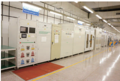
Power cell function test area
