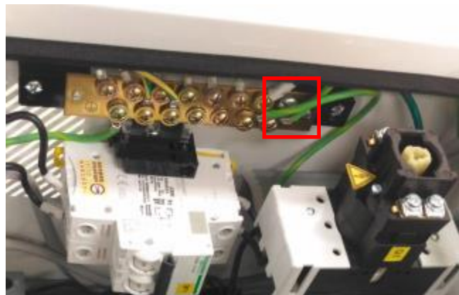
Figure8. 31 Controller grounding cable check
